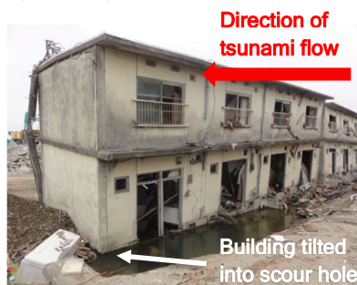
Figure 1 - Apartment block scouring at the seaward end in Yuriage, Japan due to the 2011 Tohoku tsunami (Fraser et al., 2013)
