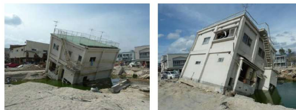
Figure 3 - The failure mode of building foundations shows tilting leading to rotation and collapsing due to a large scour hole
