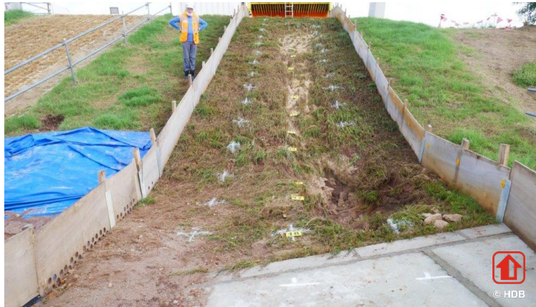
Figure 15. Test plot 8. The final situation of upper slope seen from the road after 2 hours of 50 l/s per m (a condition beyond design requirements).
