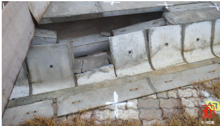
Figure 14. Test plot 7. Collapsed channel drain and large erosion hole underneath the road section, after 31 minutes of 100 l/s per m (a condition far beyond design requirements).
