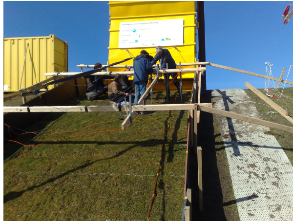
Figure 1. The overtopping simulator on the Afsluitdijk, 11 March 2009 The Netherlands. Preparation and instrumentation of the back slope for wave loading.
