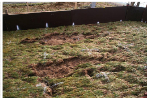
Figure 17. Various damaged locations
