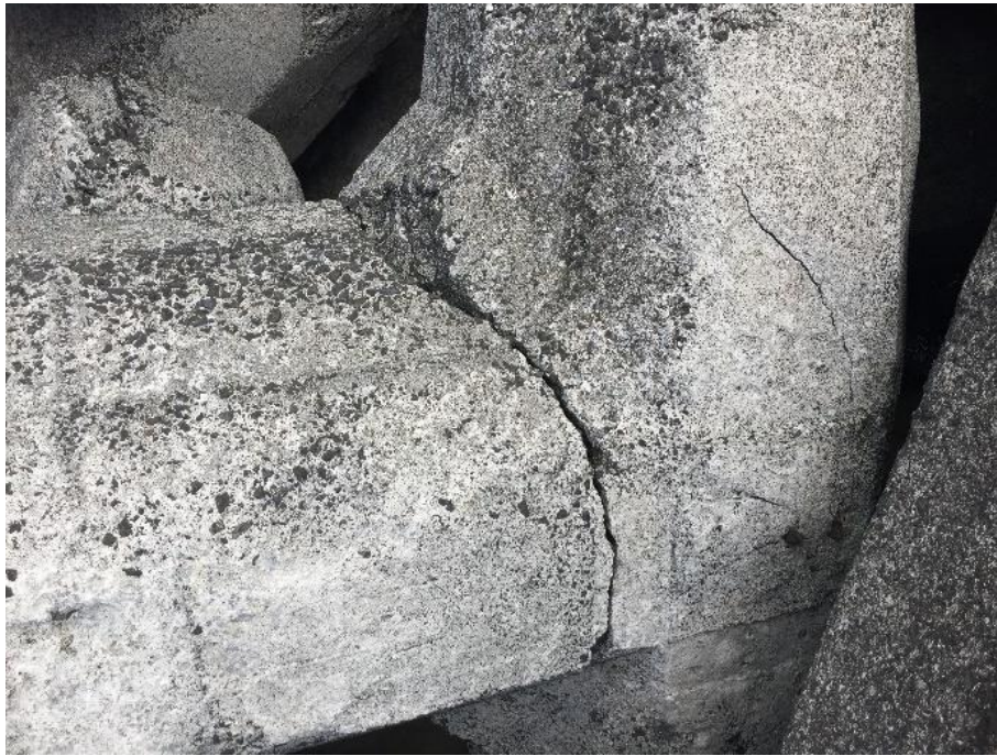
Figure 7. Broken Leg on 20t Dolos Unit
