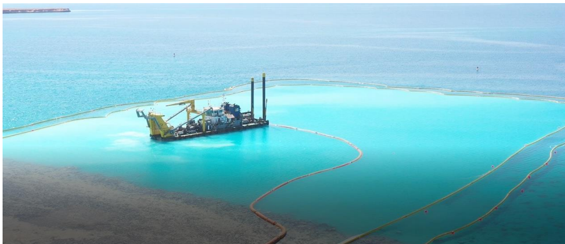
Figure 8. Sediment plume staying inside the silt screens.
