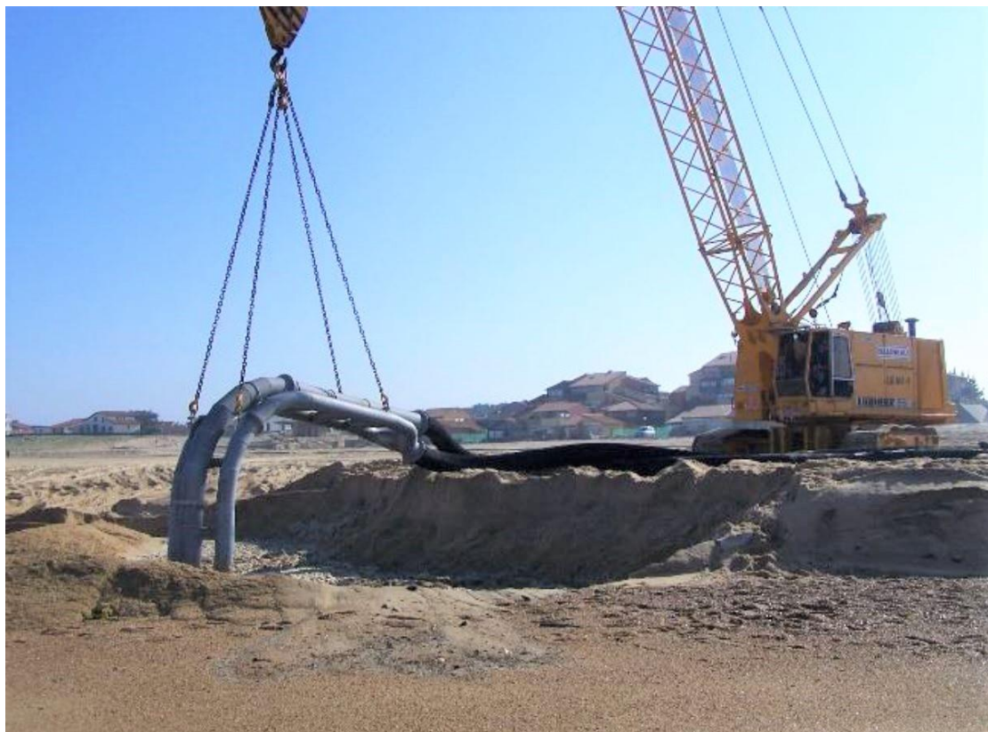
Figure 7. ASBP solutions through fixed systems: Capbreton-France – Jet Pump Arrangement and Discharge System.
