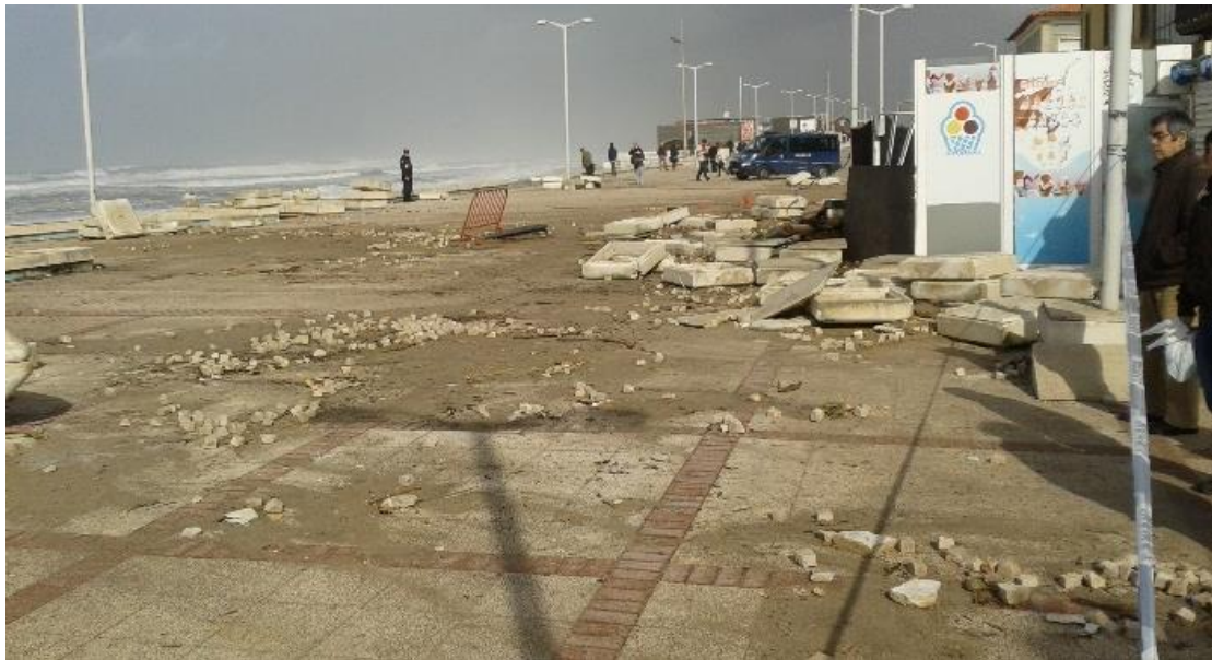
Figure 1 - Example of coastal damages registered at Furadouro beach, NW Portugal, during the 2014 storms.
