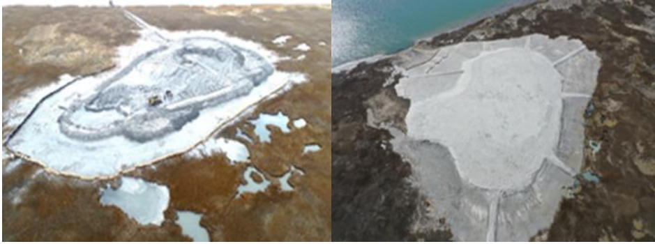
Figure 2. Sandy elevated nesting habitat at Great Flats during initial construction in 2018 (left) with placement resulting in 0.9 to 1.2m of elevation gain on the habitat area and 3-12cm of thin layer accumulation on the surrounding marsh plain. Adaptive management in 2021 (right) reestablished target elevations and early successional conditions (photos courtesy of Gary Paul).
