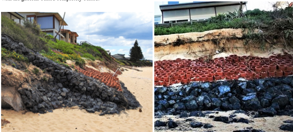
Figure 13a,b June 2016 After design storm (38 years), showing gross deformation of side and toe scour aprons. Note the depth of sand on the revetment above. Photo 13a taken 1 day after the storm subsided, photo 13a two weeks later after author arrived from overseas.
