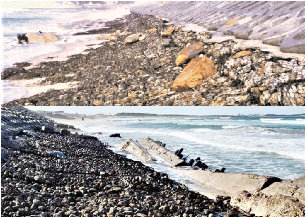
Figure 22a Gabion exposed: photo dated 14 August 1986! This is not the way to treat gabions
