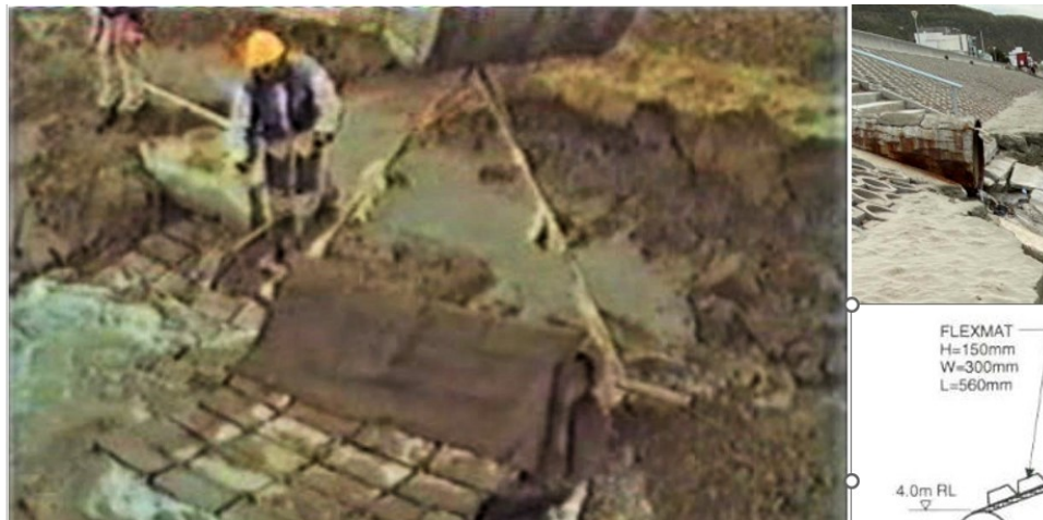
Fig 25 Flexmat – Design details, installation, and problems at a stormwater outfall.
