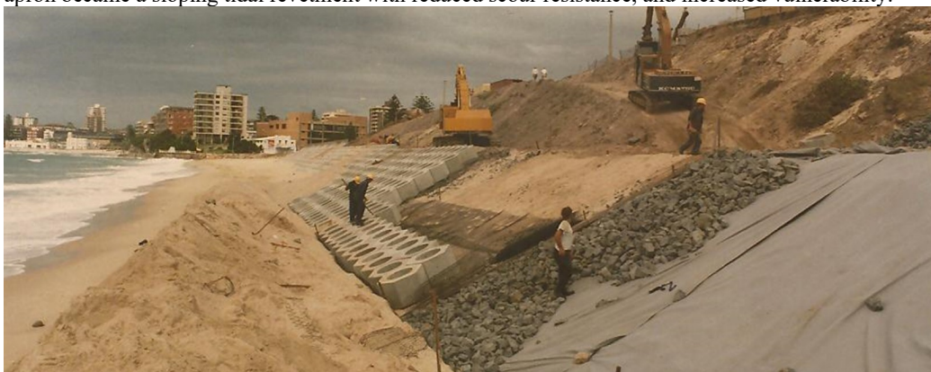
Fig 21 Cronulla seawall during construction. Underlayer blinded with sand to get an aesthetic appearance. Note the Netlon mesh, which served A) to prevent theft of underlayer and B) was to link the gabion toe to the crest wall as a tension link.
