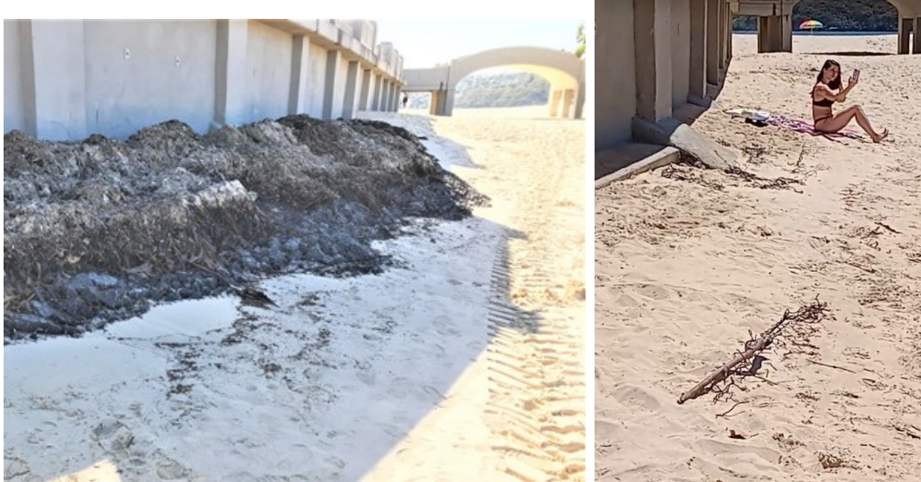
Fig 9 Exposed mattresses overlain by weed, 2021 (Photo courtesy Mosman Municipal Council), and as seen Nov 2022
