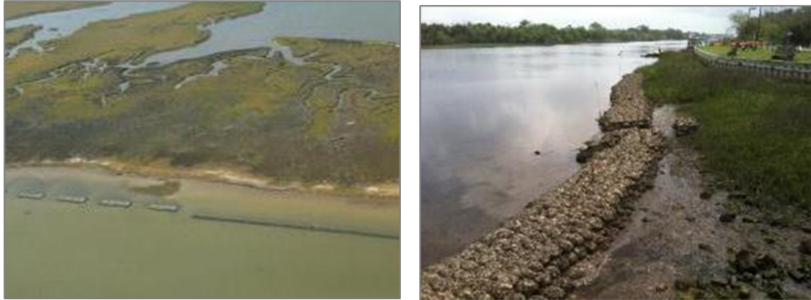
Figure 2: Examples of Type 1 Coastal NBS – Hybrid. Nearshore reefs to reduce marsh erosion. Photo credits: The Nature Conservancy. Right image. Oyster reefs constructed from bags of oyster shells
