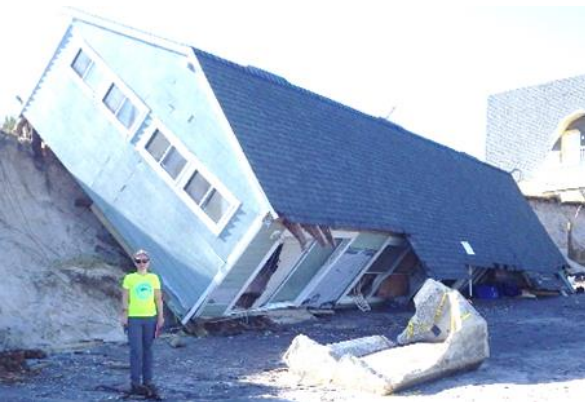
Fig. 2. - Post-Hurricane Irma photograph of slab-on-grade house destroyed by bluff erosion (R-110).
