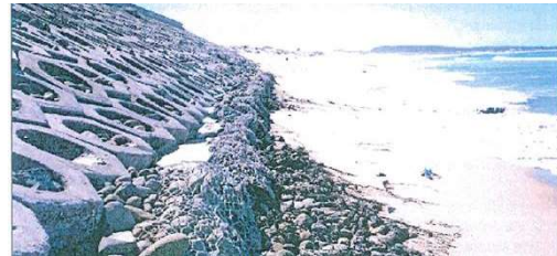
Figure 3: Original Prince Street seawall with failed rock gabion mattress
