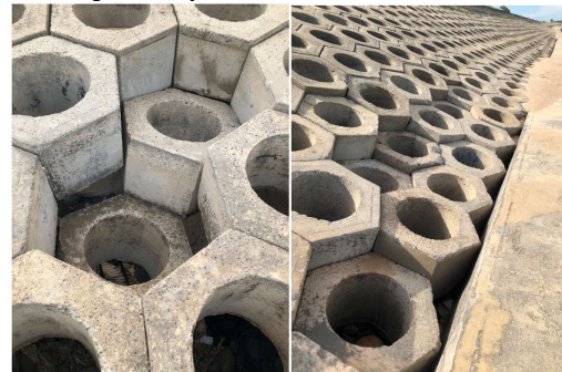
Figure 4 Undermined Seabee units at Prince Street Seawall, 2020
