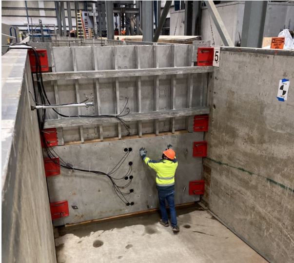
Figure 3 - Leaside of the vertical aluminum wall placed in the flume. Red clips fix the wall to the flume concrete sides. Note the location of the pressure gauges installed along the centerline.
