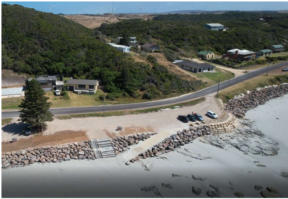
Figure 3 - Seawall texture and block placement - Turtle shell, random block placement and blocks
