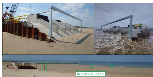
Figure 2 - The artificial dike and intertidal poles at low tide (top left and bottom) and high tide (top right)
