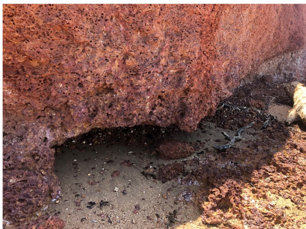
Figure 4 - Severe notch erosion observed at the base of the cliff prior to commencement of works
