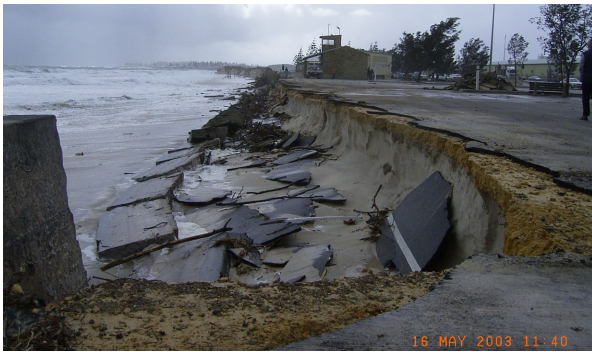
Figure 1 - Major Erosion at Port Beach in May 2003
