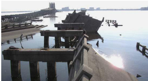
Figure 2. Damage to the U.S. 90 Biloxi Bay Bridge caused by Hurricane Katrina.
