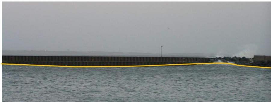
Figure 3. Severe overtopping of the breakwater just south of the harbour entrance (upper figure) and wave disturbance inside the harbour basin.
