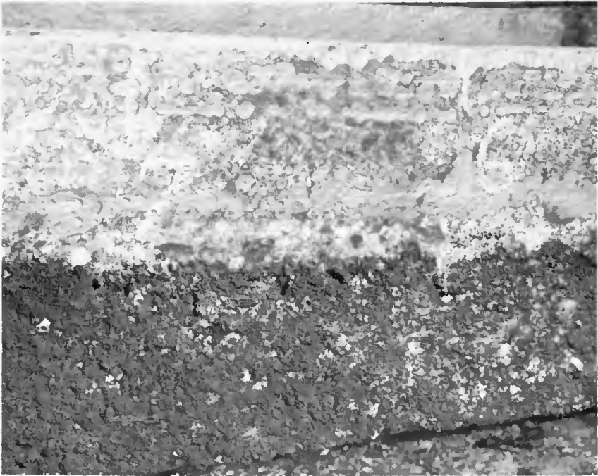
Fig. 1. Corrosion pattern on unencased pile.
