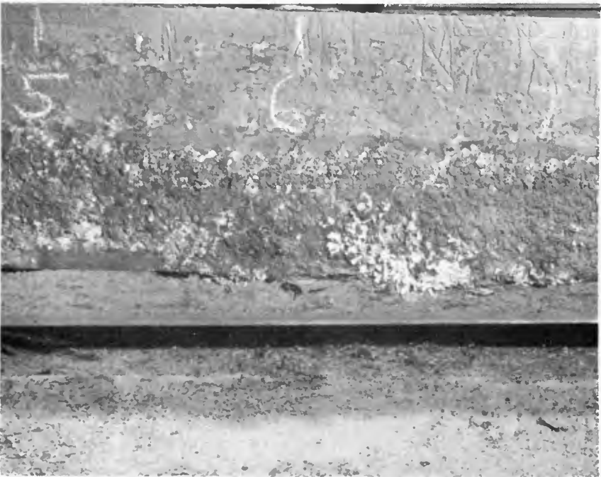
Fig. 2. Corrosion pattern on encased pile.
