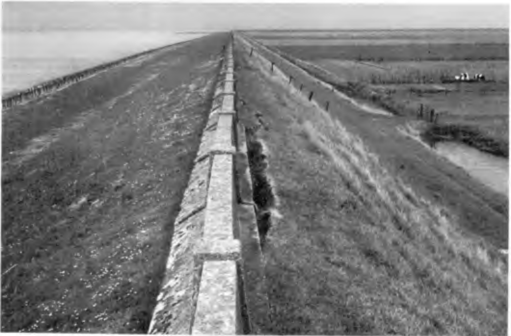
Fig. 12. The first stage of the attack. The fissure on the crest is caused by the strong pressure difference in the ground water.
