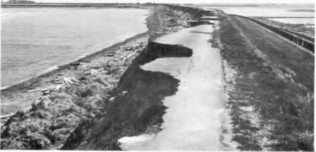
Fig. 11. A damaged dike. The sea is on the right and the land was to the left. Damage occurred at the inner side.
