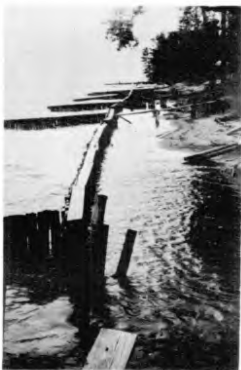
Fig. 2. An example of ineffective sea wall and groin construction.
