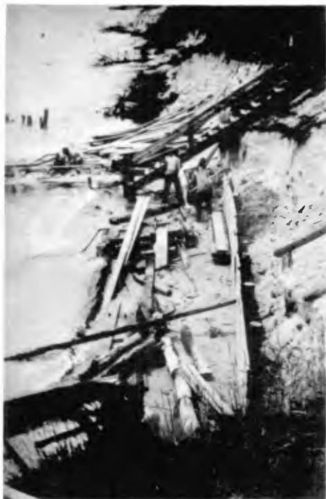
Fig. 1. An example of inadequate sea wall construction.
