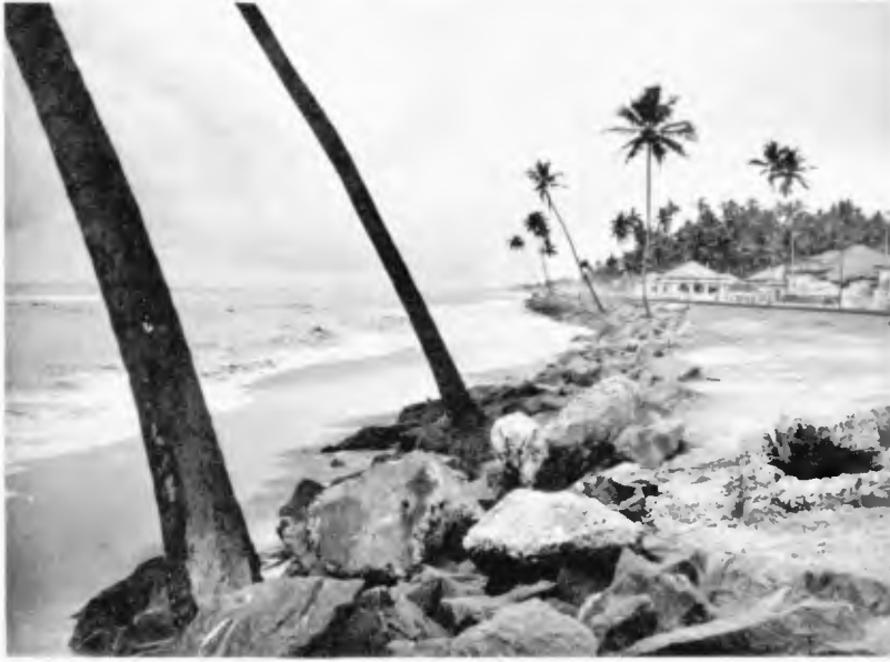
Fig. 4. Coast lined with rock stones supported at the bottom by a coral reef.
