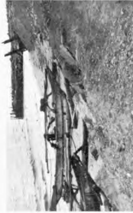
Fig. 2. Southern jetty at Wellawatta Canal outlet in the process of construction. Note the absence of a sandy beach.
