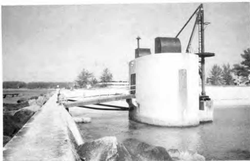
Lake Worth sand bypass plant, Palm Beach, Florida. Photo courtesy of Billy L. Edge.
