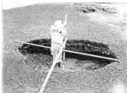
Photo 1(a) A large hole formed behind a seawall.
