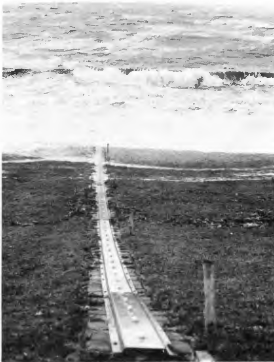
Fig. 7 Waves acting on the dyke at Stintek location during a storm surge
