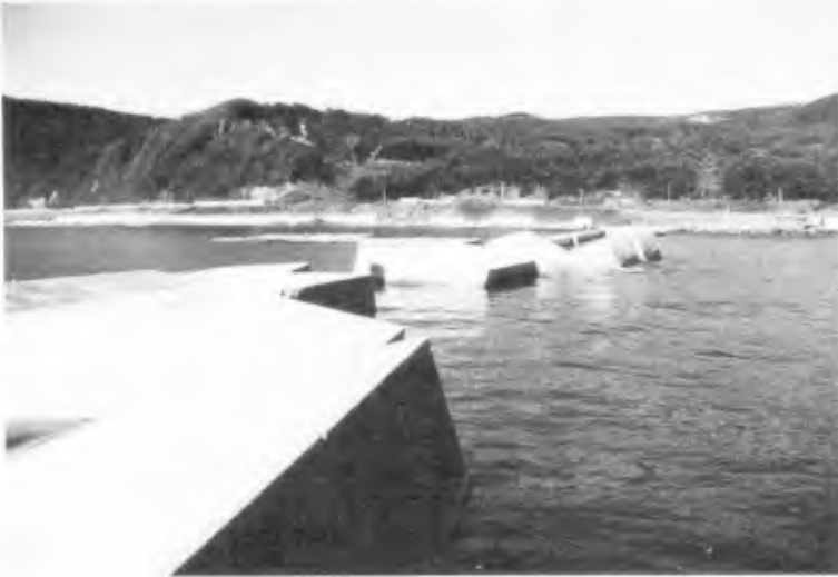
Photo 1 Damaged composite breakwater(1993 Okushiri Port )
