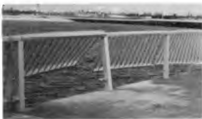
Figure 1 Photograph of damaged breakwater handrails
