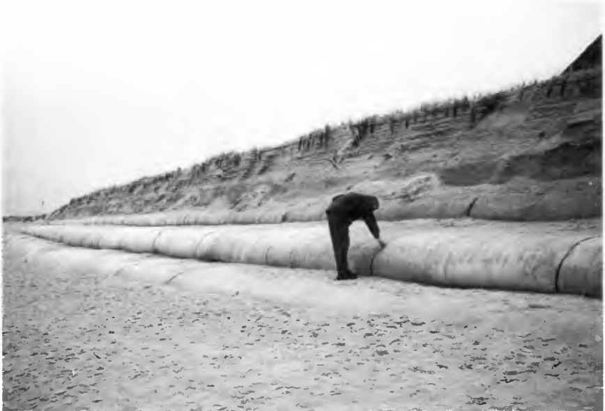
Fig. 11 Uncovered geotextile membrane in front of a dune after called in action during a storm surge (photo: Raudkivi, 1994)
