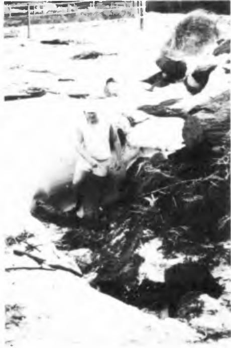
Figure 11: Scour hole formed on the beach next to the southern breakwater on 22-6-89
