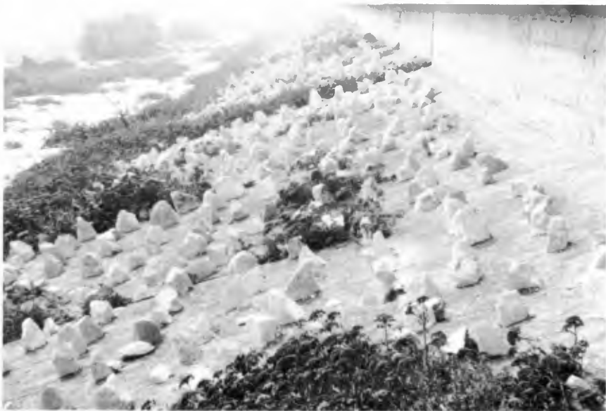
Photo 1-2 Views of the existing murazzi at Pellestrina (in some areas with macro-roughness elements)
