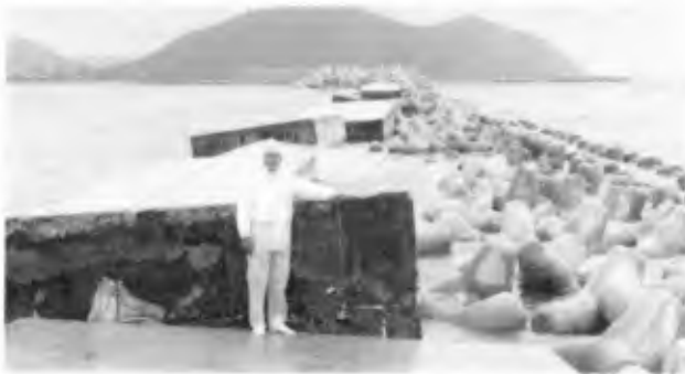
Photo. 1 Damaged breakwater due to Typhoon high waves
