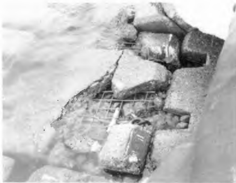
PHOTO 4: BLOCK BREAKAGE CAUSED BY ICE IMPACT
