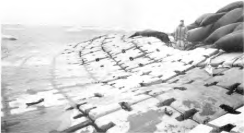
PHOTO 2: POST-STORM CONDITION, OBLIQUE ANGLE OF WAVE INCIDENCE
