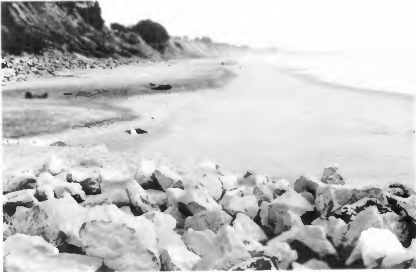
Figure 9. Localized scour adjacent to downcoast end of seawall.
