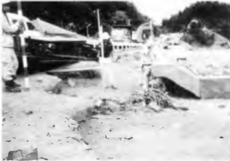
Photo. -2 Destroyed seawall and road due to storm surges (Sosu coast, Typhoon T8613)
