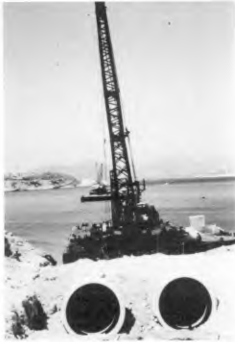
ON-SHORE TERMINUS OF SIPHON PIPES
