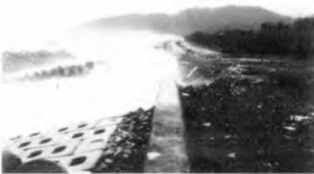
Photo 12. Heavy waves overtopped the crown of the experimental seawall, on the 20th December 1986.
