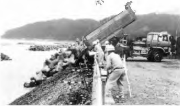
Photo 9. Filling of sand and gravel, which were diverted from the dredging of Miyazaki fishing port, located 4 km away from the site ( cf. Fig.7 ).
