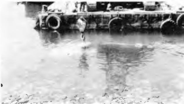
Photo 10. Setting the Lotus-Uniblock on the rubble stone. The lowest block were set at -3.3 m water depth.
