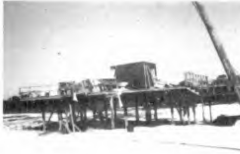
Photograph of structure foundation that is essentially undamaged. The wind forces probably tore the structure from the foundation leaving the floor attached to the piles. Most of this damage was caused by the wind forces.
