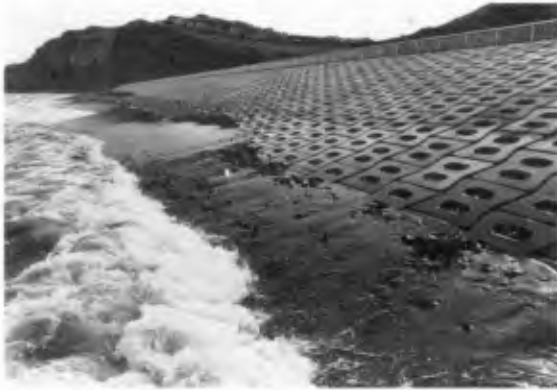
Photo.8 Gravel are left on the toe of the seawall
