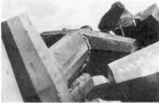
FIG.4 TYPICAL DOLOS BREAKAGE (6-TON UNITS AT STA 119+25)
