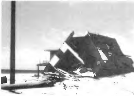
Photographs of structure torn from its foundation. Wave and wind loads probably caused the damage.
