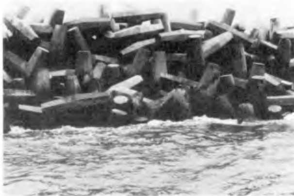
FIG.5 TYPICAL DOLOS BREAKAGE (4-TON UNITS AT STA 128+50)
