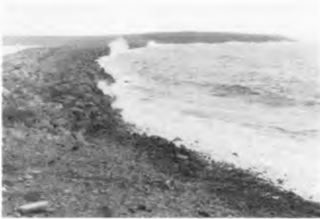
Figure 8. Codroy Breakwater After Construction. Breakwater Extends From Beach (in foreground) to an island
