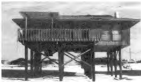
Photograph of "X" braced structure that has received very little damage at ground level. Erosion of soils was approximately three feet.
