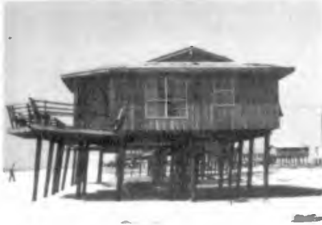
Photograph of structure that is essentially undamaged except for leaning piles and obliterated stairs. The leaning piles were probably caused by a combination of excess wind loading and loss of soil resistance due to erosion of about two feet of sands. The obliteration of the stairs was probably caused by wave forces.
