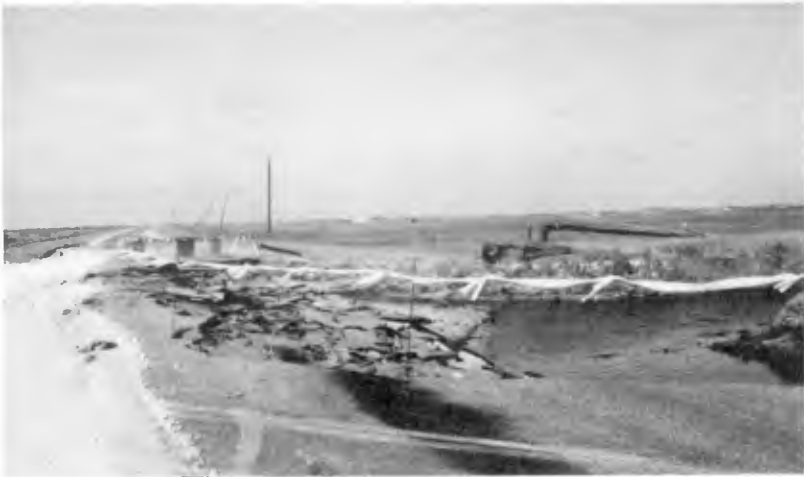
Figure 6. Landward end of a Follets Island cut showing undercutting of road pavement.
