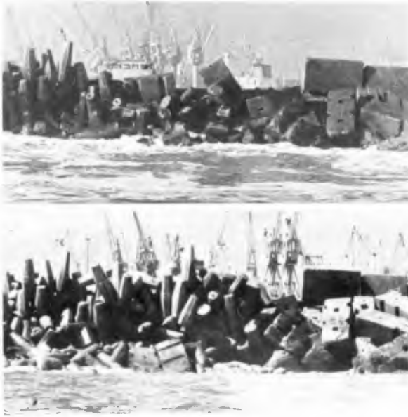
Figure 2 Loss of dolosse at section P10
