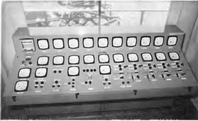
View of Panel in Control Cabin.
