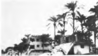
Fig. 3. Summer houses at El Arish, N. Sinai. The collapse was a result of the sand deficit caused by quarrying of beach sand ("Zifzif") nearby.
