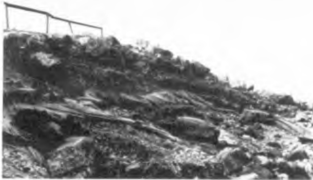
FIG. 7. FAILURE OF PANELS 3 AND 4, JANUARY 1978.
