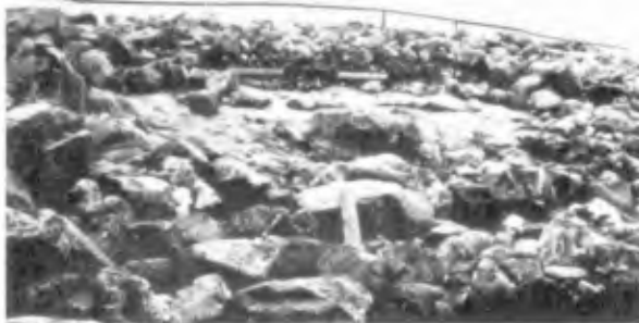
FIG. 6. FAILURE OF PANEL 1, NOVEMBER 1975.
