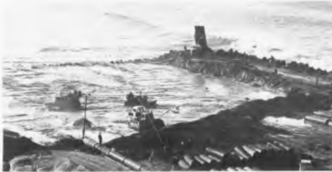
ill. 13. Protruding stone wall shifted forward and acting as knife-edge. Note the size of the breaking waves.
