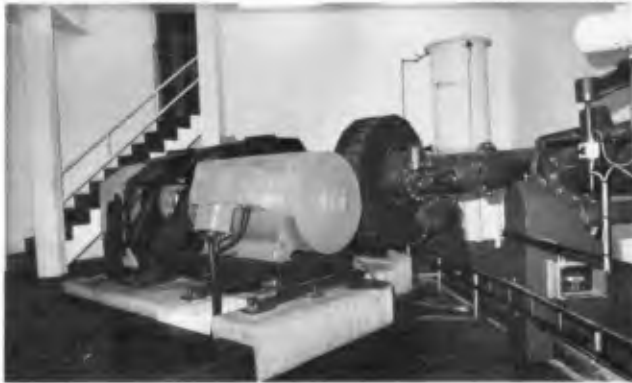
Typical Booster Motor and Pump Set.
