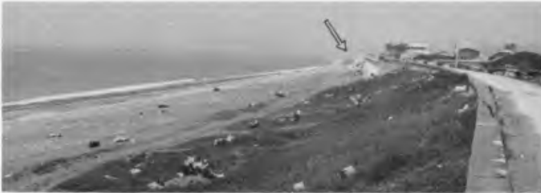
Fig.26 Vertical seadike was partially destroyed
