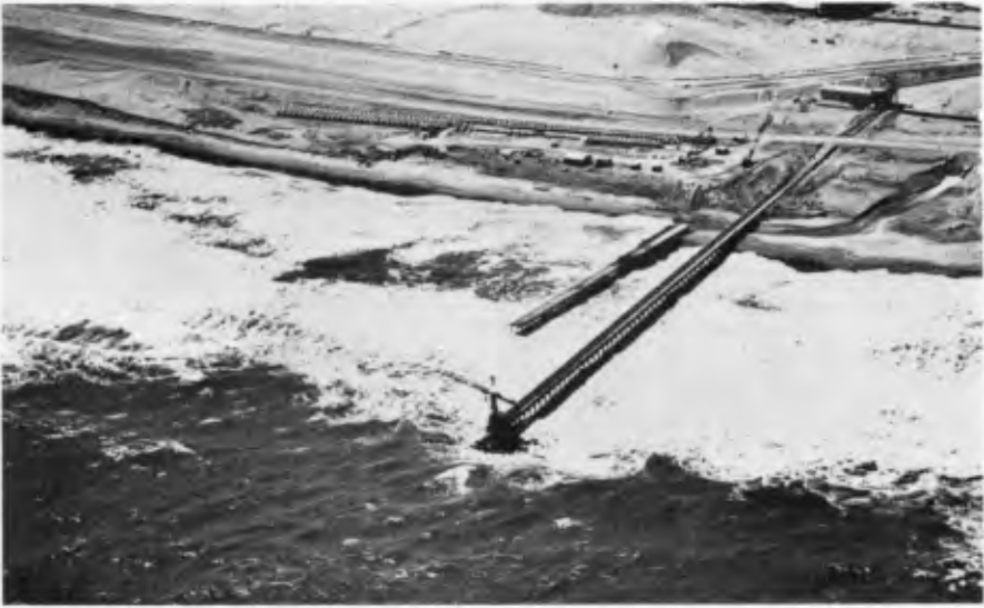
FIG. 6 HEAVY SURF POUNDING THE STRUCTURE
