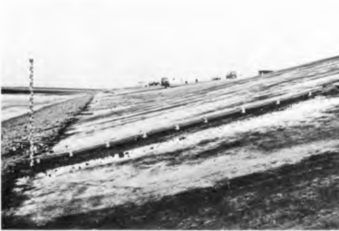
Fig. 7 Asphalt covered sand dyke of the Eider storm-surge barrage with test section (pressure cells before fitted in the asphalt cover)
