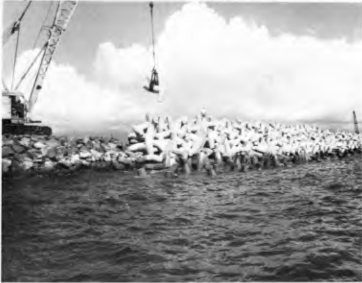
FIGURE 13 Crane placing dolos - Showing a view from ocean of completed dolosse armor.
