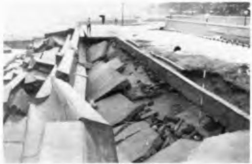
Fig.10 In January 1961, the stepped face seawall had been partly destroyed by the winter strong wave force. Waves had scoured beach at the foot of the seawall, and the body of the seawall had been scattered. The seawall had been reconstructed at once.
