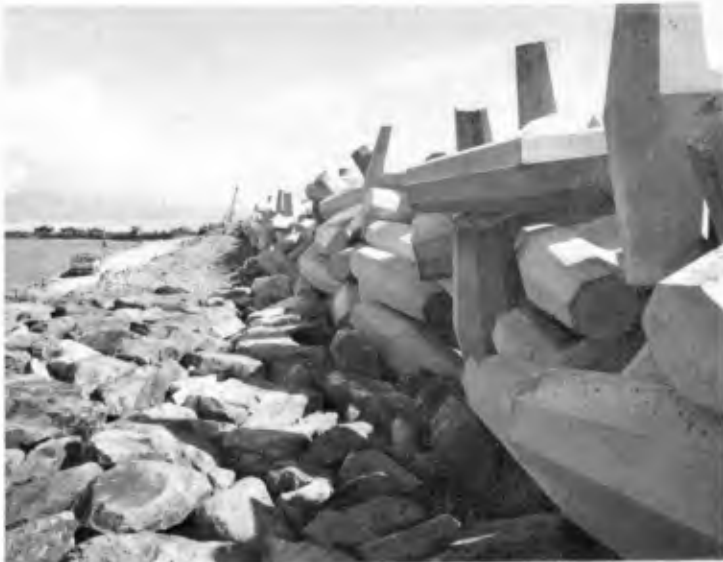
FIGURE 14 View along backside of structure showing dolosse in place prior to placing back up armor stone.
