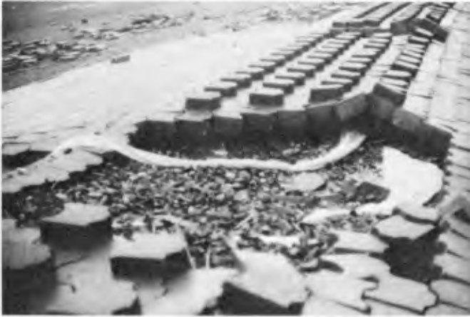
Fig. 12 Typical damage of stone revetments due to wave impacts
