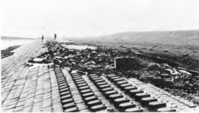
Fig. 3 Damage of a stone revetment due to wave impacts
