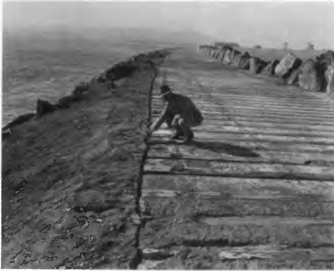
FIGURE 15. Beginning of slope separation failure--Humboldt Harbor and Bay South Jetty.
