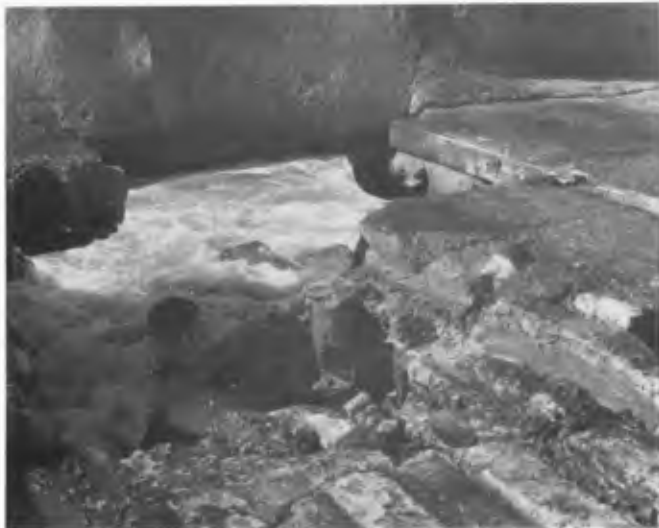
FIGURE 14. Advanced stages of uplift pressure failure--Humboldt Harbor and Bay North Jetty.
