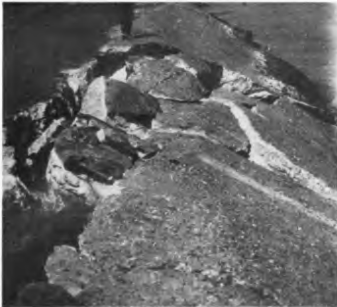
FIGURE 16. Advanced slope separation failure--Humboldt Harbor and Bay South Jetty.
