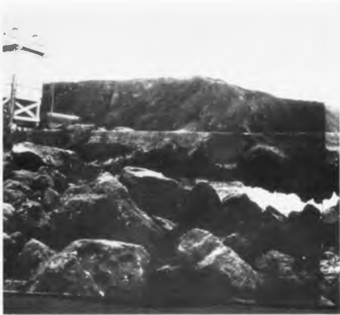
FIGURE 24. Failure of rigid structure due to undermining--Noyo River and Harbor North Wall and Jetty.
