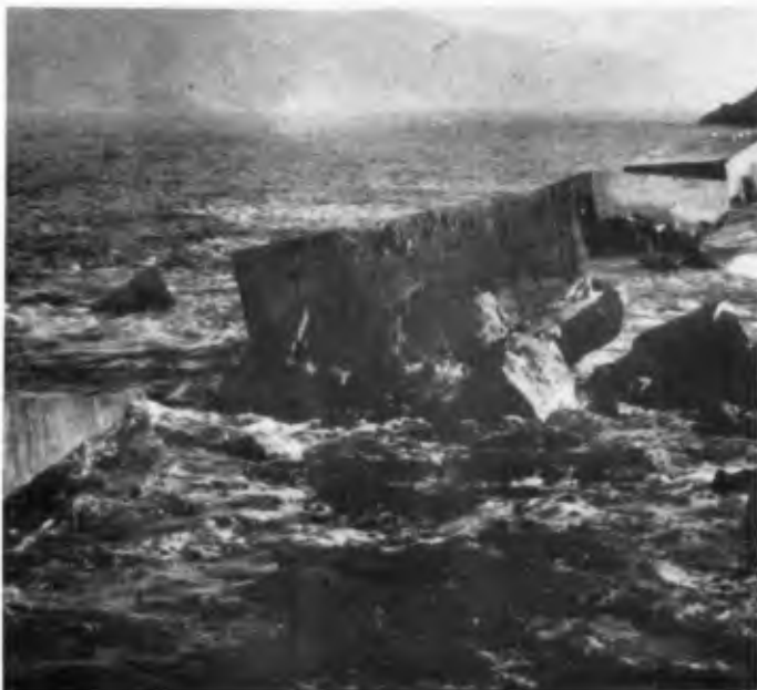
FIGURE 4. Damaged original extension of Crescent City Outer Breakwater-- viewed from Station 36+70 with Round Rock in distance (upper right).
