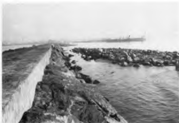
FIGURE 10. Wave trench resulting from the overtopping shown on Fig. 9-- Crescent City Outer Breakwater.
