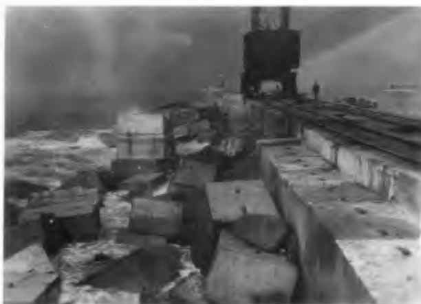
FIGURE 19. 20-ton pre-cast concrete blocks circa 1932--seaward face of Humboldt Harbor and Bay South Jetty.
