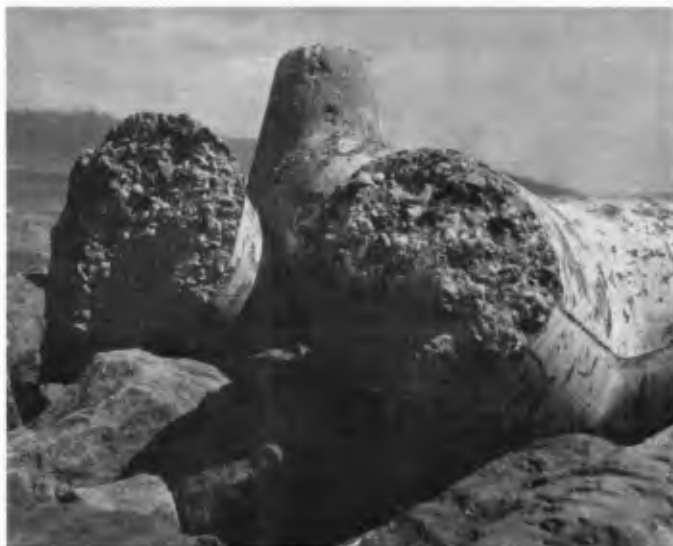
FIGURE 8. Tetrapod damaged by storm wave attack on repaired area shown on Fig.6.
