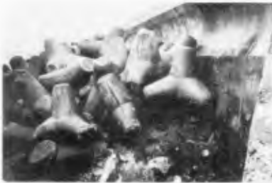
Fig. 17 - New damages at North breakwater
