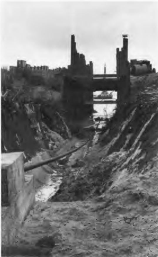
Pipe-pulling through the dune trench in May 1973. Note bitumen spray on trench sides.
