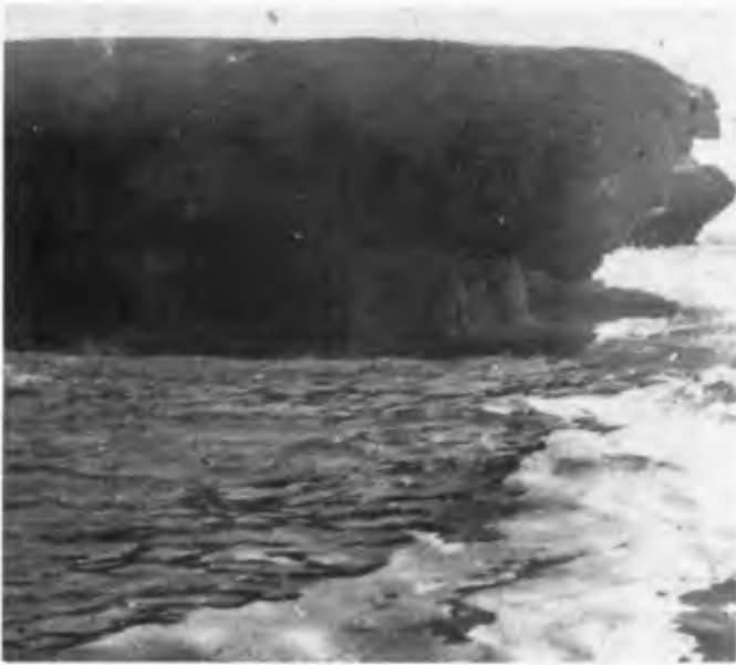
FIGURE 17. Displacement of ring dike and lack of concrete penetration--seaward head of Humboldt Harbor and Bay North Jetty.
