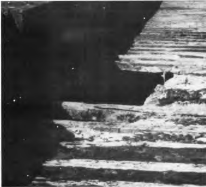
FIGURE 13. Uplift pressure failure--Humboldt Harbor and Bay North Jetty.
