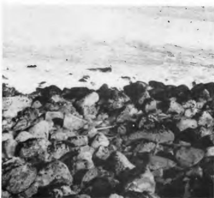
FIGURE 20. Stones displaced from seaward head of Humboldt Harbor and Bay North Jetty showing extensive rounding due to impact and abrasion.
