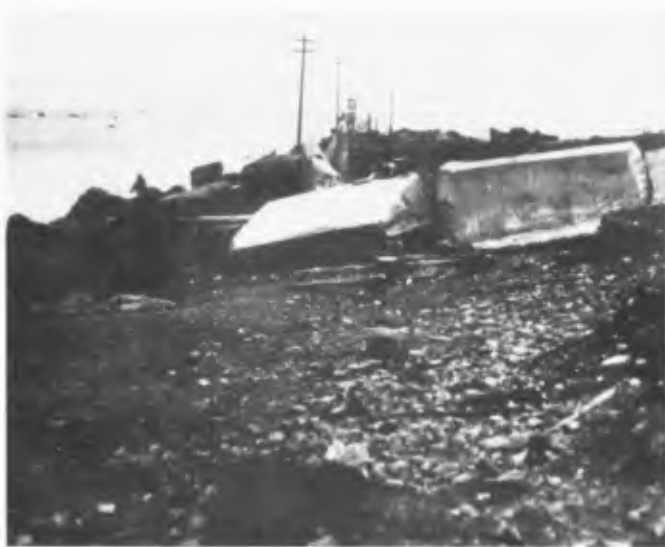
FIGURE 25. Advanced failure of rigid structure due to undermining--Noyo River and Harbor North Wall and Jetty.
