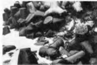
Fig. 18 - New damages at North breakwater
