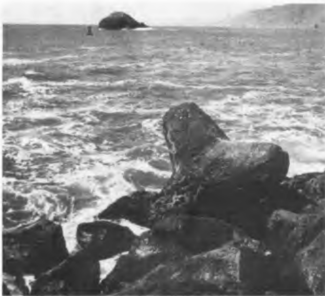
FIGURE 7. Storm wave displacement of originally submerged tetrapod from repaired area shown on Fig.6.
