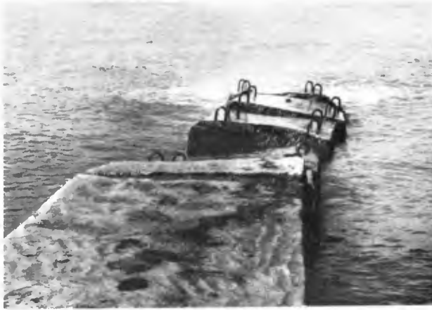
Fig. 1. Deformation of the conventional groin.
