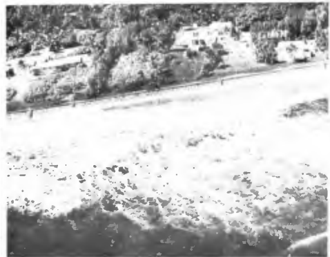
Fig. 37. Interlocking block revetment on Jupiter Island under heavy wave attack (Bruun and Manohar, 1963)
