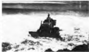
Fig. 54. Bulldozer operation at Deerfield Beach, Fla., following the March 1962 storm (Bruun and Purpura, 1963)
