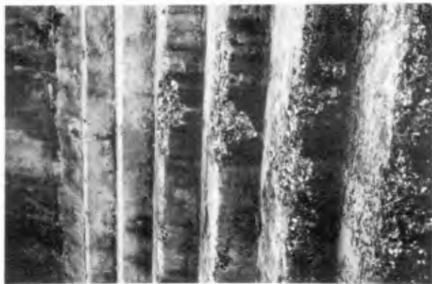
Plate VI Spalling of stepped concrete apron possibly initiated by crystal growth in hair cracks
