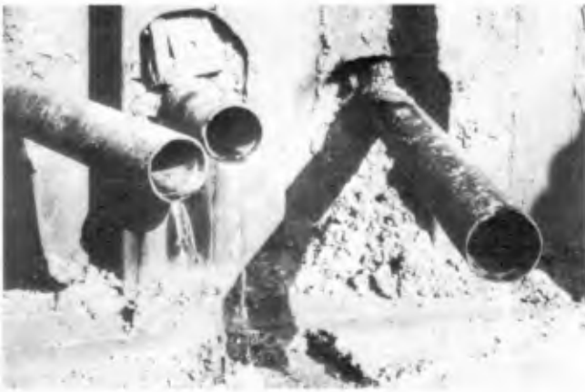
Fig.2: Auger-bored inclined drains lined with pitch fibre pipes ready for connection to the collecting toe drain.
