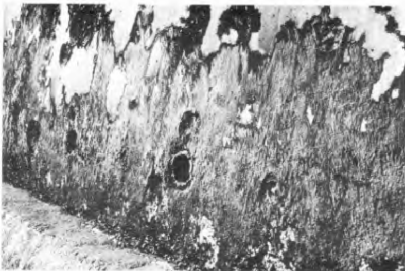
Plate I - Surface deterioration possibly due to seaweed growth
