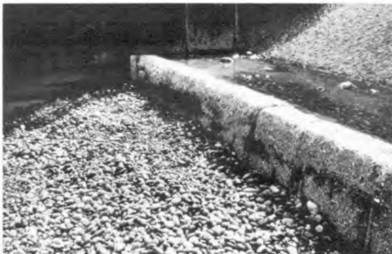
Plate IV - Sea Wall at Sheringham constructed with precast concrete retaining wall units as permanent formwork
