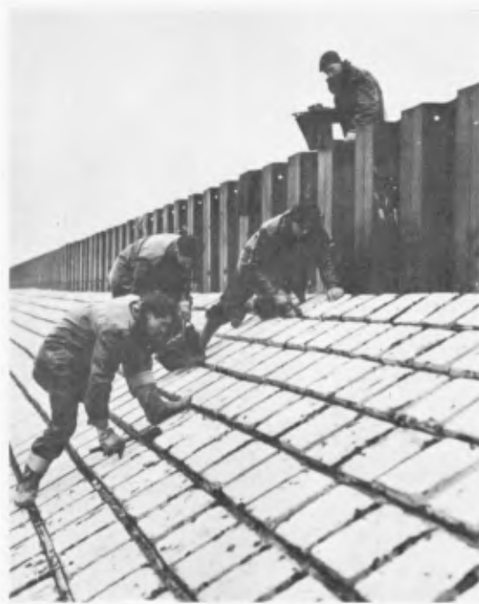
Photo 2. Asphalt jointing (Photo by courtesy of the Chief Engineer - Essex River Board).
