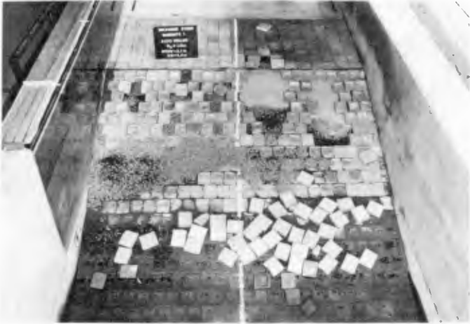
Fig. 14 Damaged revetment I and II after wave attack
