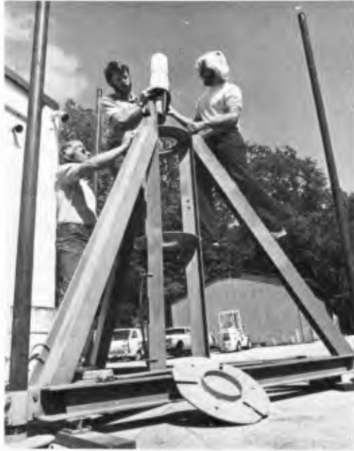
Figure 3 Dry run of instrument installation in underwater tripod mount. Note top retaining plate in foreground and anchoring pipes at apexes.
