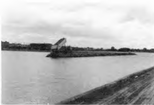
Figure 10. North Bay Breakwater During Construction. Construction Required Only Trucks and a Bulldozer
