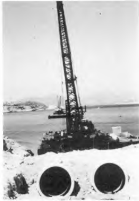
ON-SHORE TERMINUS OF SIPHON PIPES
