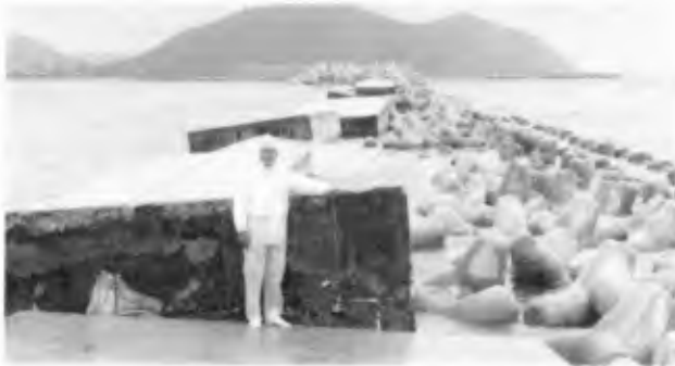
Photo. 1 Damaged breakwater due to Typhoon high waves
