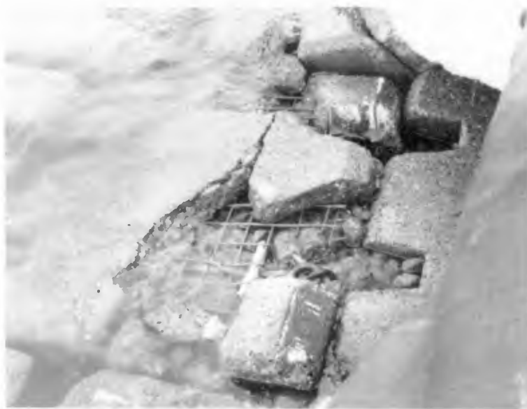
PHOTO 4: BLOCK BREAKAGE CAUSED BY ICE IMPACT
