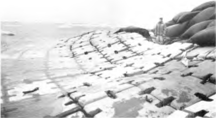
PHOTO 2: POST-STORM CONDITION, OBLIQUE ANGLE OF WAVE INCIDENCE
