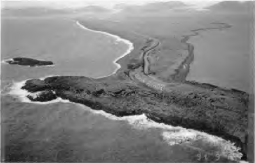
Figure 5. Construction of the shore protection on the South Barrier. The alignment of the shore protection is set according to the maximum known scouring from the entrance
