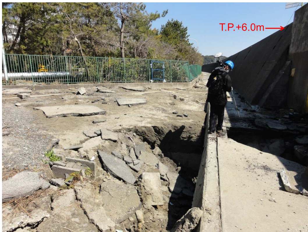
Figure 5. Intact parapet, apron concrete broken and land scoured by overflowed tsunami in Power Plant District. (March 25, 2011)
