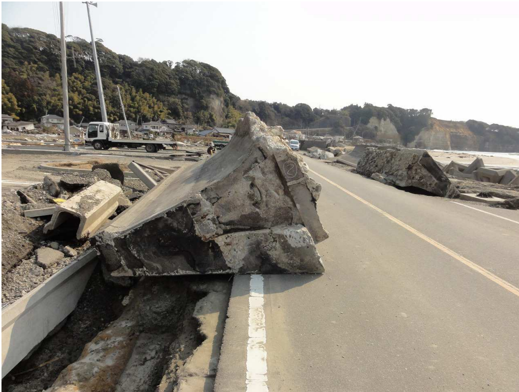
Figure 7. Broken and moved parapet of a seawall in Iwama District (March 25, 2011)
