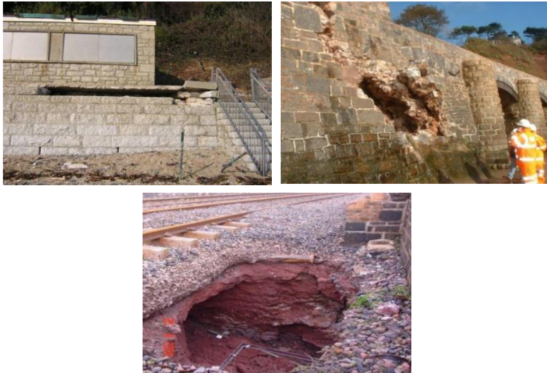
Figure 2. Damage due to wave overtopping to the seawall (top panels) and damage due to wave overtopping and flooding to the South-West main railway line (bottom panel).
