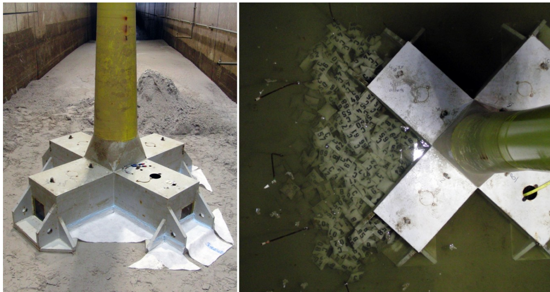
Figure 4. Foundation with installed fleece for Variant 2 (left) and foundation during installation phase of the scour protection system (right).
