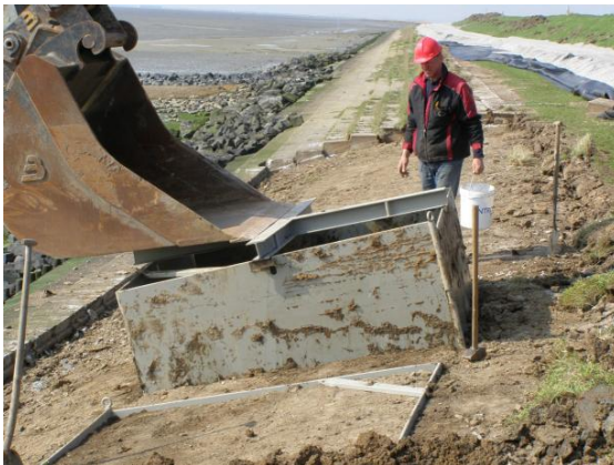
Figure 8, Pushing the steel box without bottom into the clay with hydraulic crane
