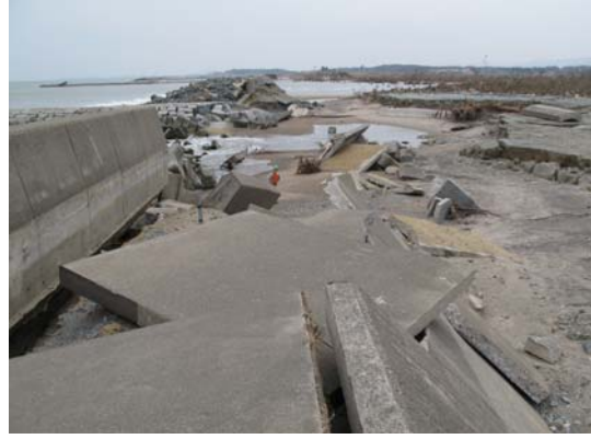
Photo 19. Breaking of the top and landside concrete slabs, southern Yamamoto Coast.
