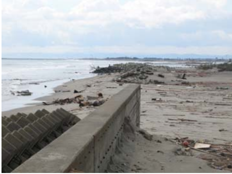
Photo 6. Overlook the breach point from the north photographed on March 26, 2011
