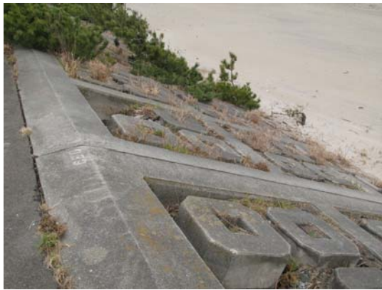
Photo 20. Seaside armor blocks of the levee, northern Yamamoto coast.
