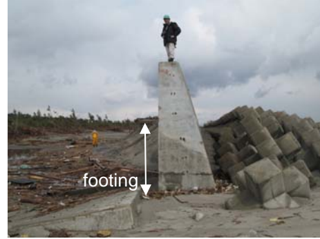
Photo 7. Overlook the concrete levee from the breach point
