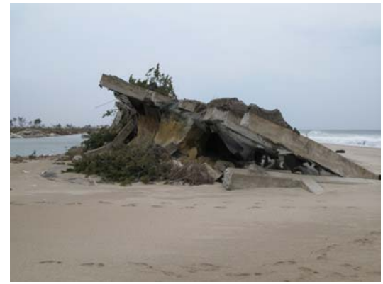
Photo 23. Destructive erosion of the levee at the break pint.
