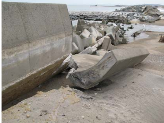
Photo 18. Breaking of recurved parapet, southern Yamamoto Coast.
