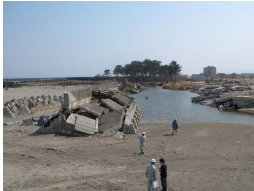
Photo 12. Broken coastal levee and newly formed channel
