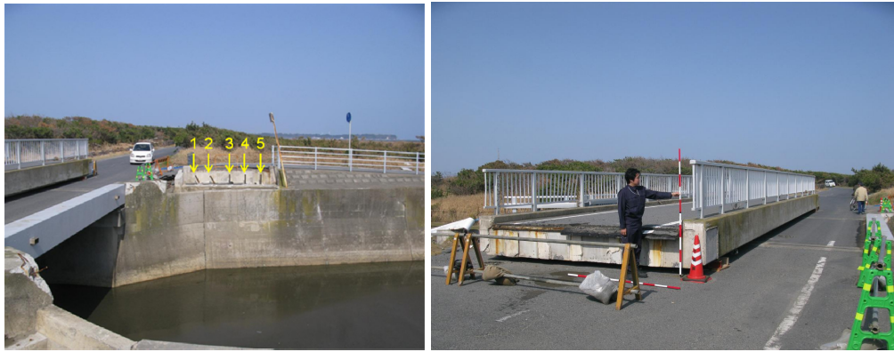
Figure 2. Right photo shows the flooded slab and left photo also shows the deformations of anchor bars.
